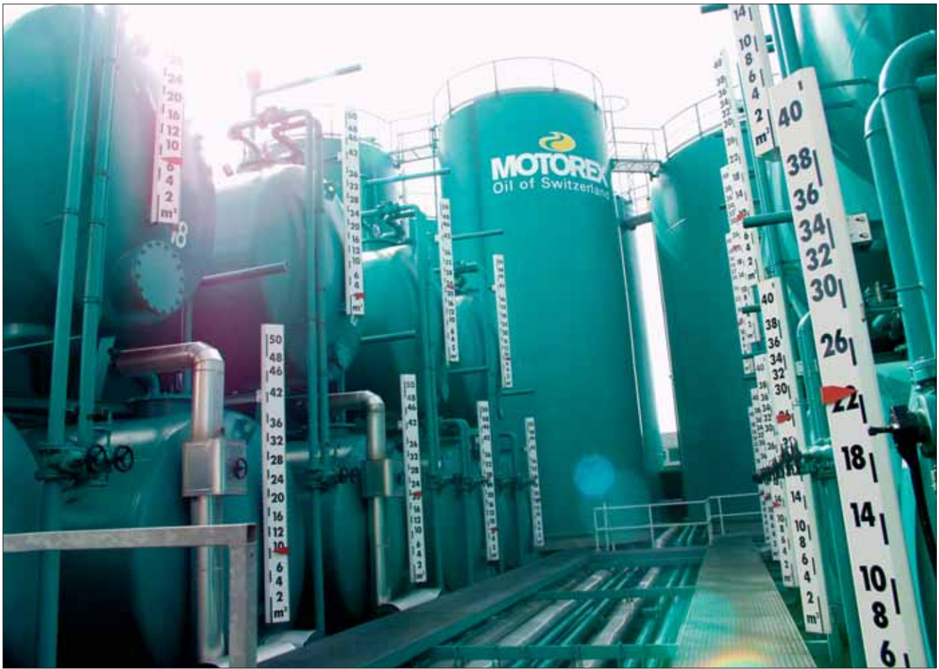
View of the tanks at Motorex: For each type of application, the quality of the basic oil is selected with care. (Photo: Motorex)
