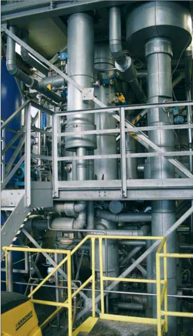
This is not a view inside a chemical plant but the three-level vacuum evaporator which turns contaminated water into very clean water.
